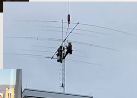
New ARDC-Funded W3USR HF Antennas
